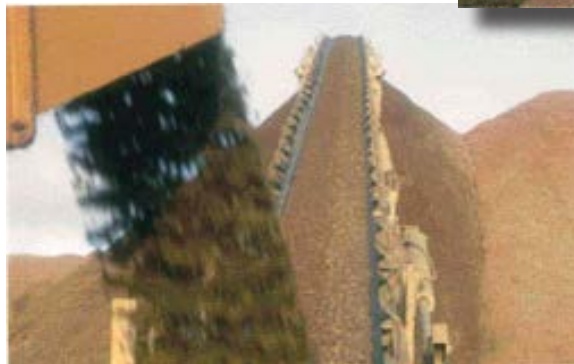
Below, the discharge conveyor from a crushing plant is in the foreground. Notice how badly segregated the material is as it is carried up to the stockpile on a belt stacker. This invariably leads to problems illustrated in the two photos to the right.
