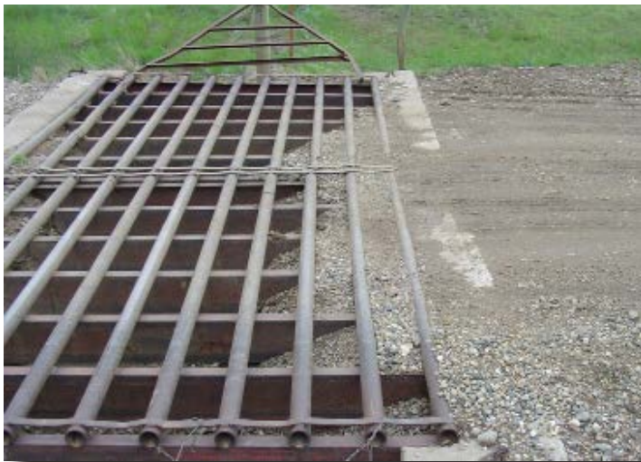
Care must be taken not to spill gravel into the cattle guard. Poor quality gravel with too much loose aggregate aggravates the problem of material spilling into the cavity spill gravel into the cattle guard.
