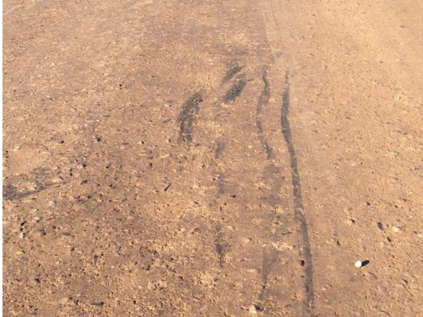
Outstanding record of performance on the same magnesium chloride stabilized road with a skid mark clearly evident.
