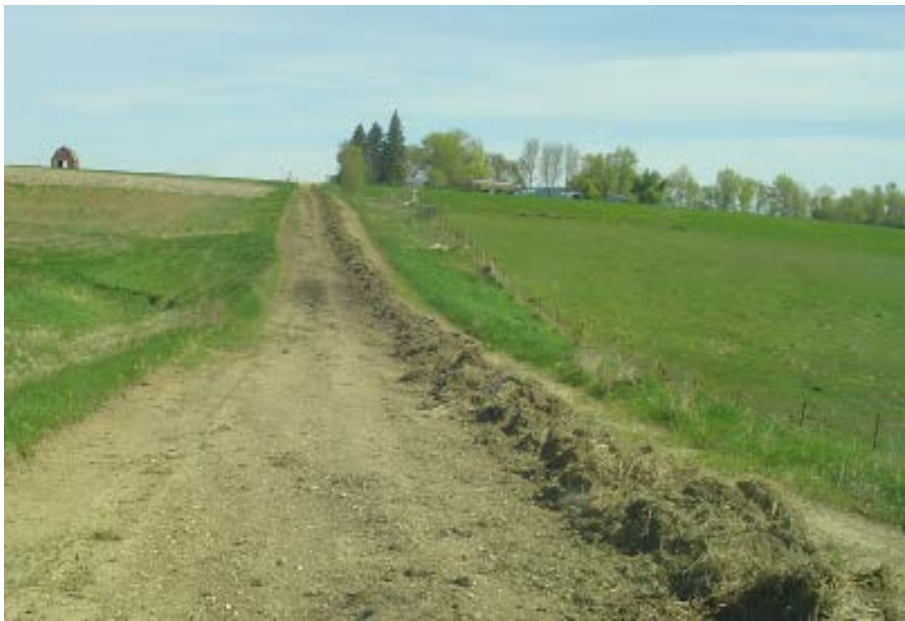
This windrow is excessive and should never be left on the roadway. It is a bad practice even on a very low volume road. Multiple passes should have been made with the grader to work the vegetation out of the windrow or other mechanical means such as a disk should have been used to break up the chunks of sod so more material could be spread on the roadway.
