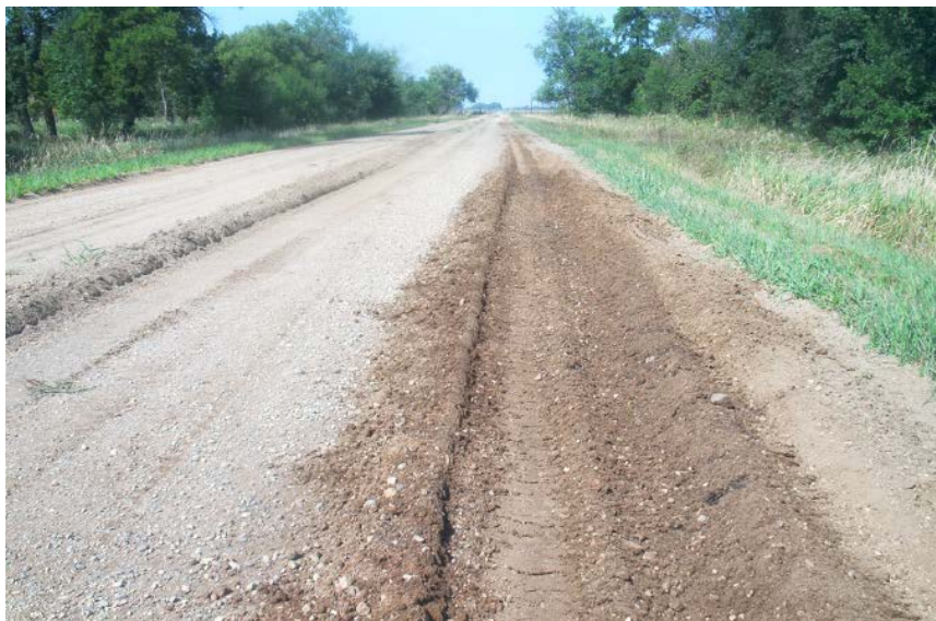
Example of road that carries heavy trucks and begins to fail in any wet condition or during spring thaw in cold regions.
