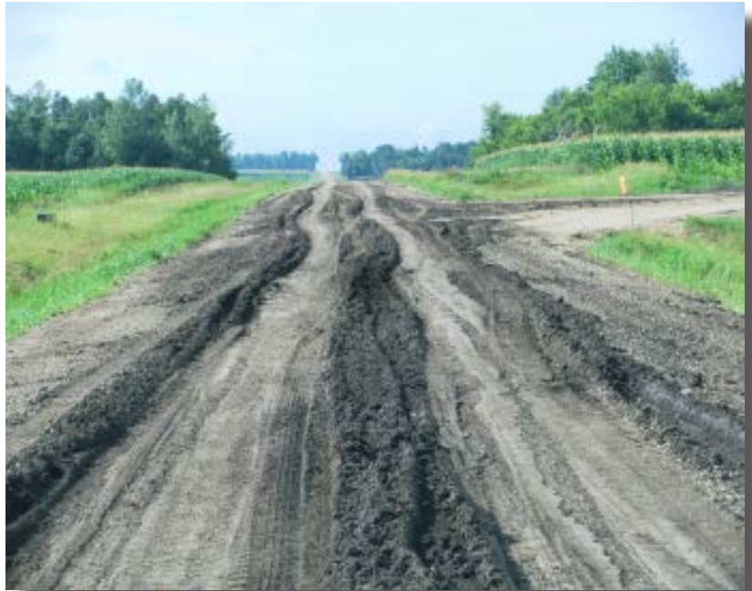
This road has been damaged by a heavy haul. Reshaping the entire road surface is required before new gravel is placed.
